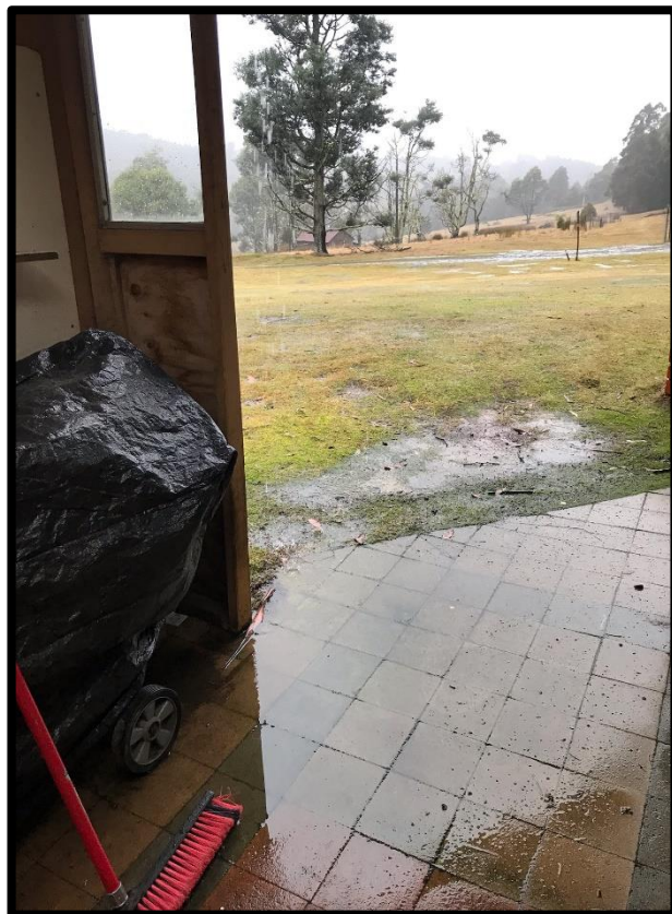
Water needing to be swept out of the BBQ area (KM)
